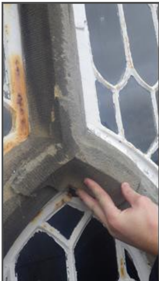
Window stone failure
